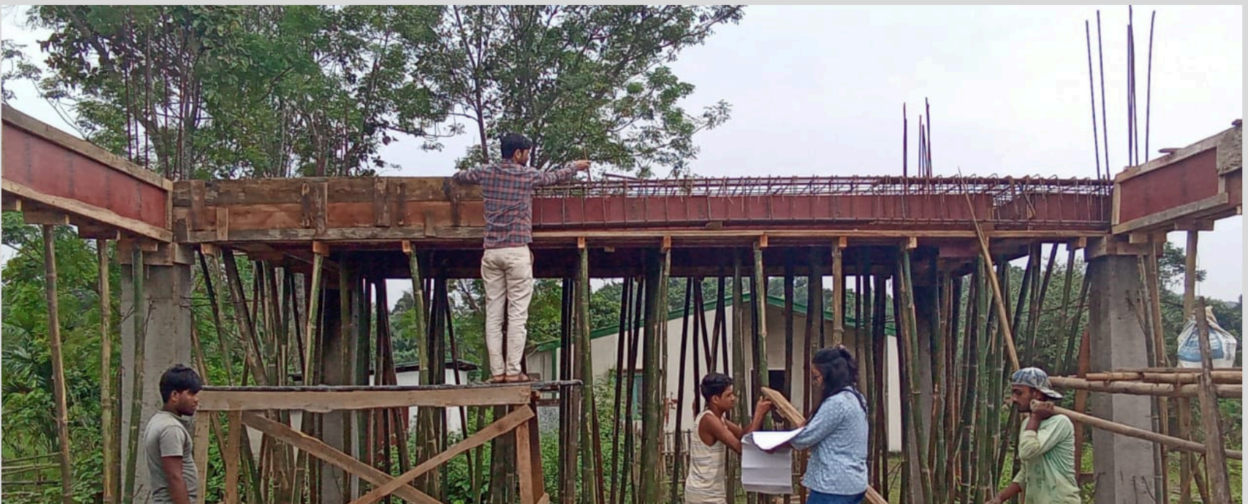
Update on the progress of Phase II construction work at Nayapara village, within the Tikrikilla BPMU, West Garo Hills.
